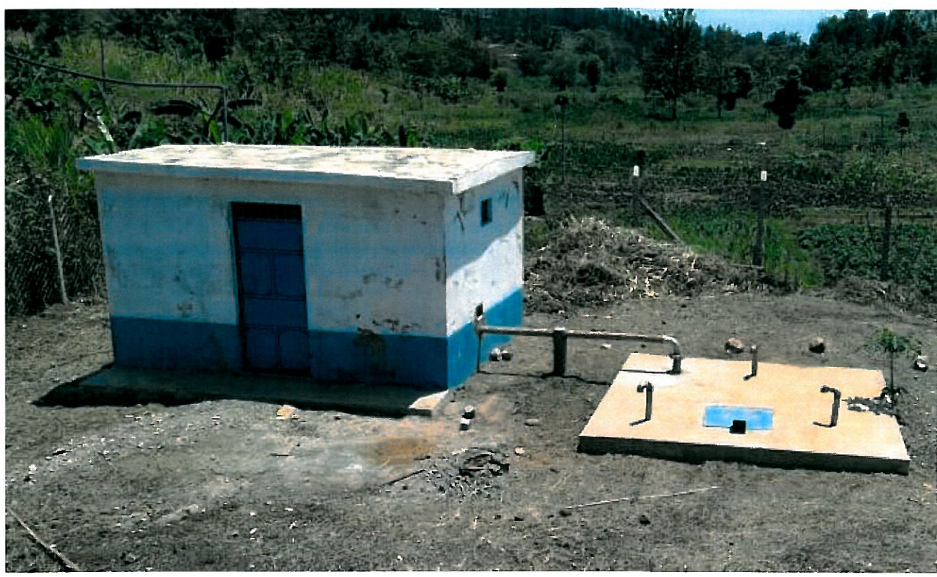
Pump house & swamp tank
