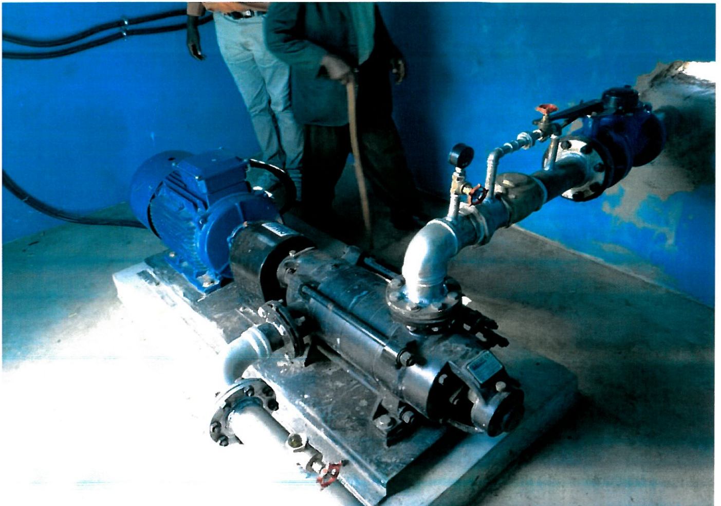
Complete Water Pump with accessories
