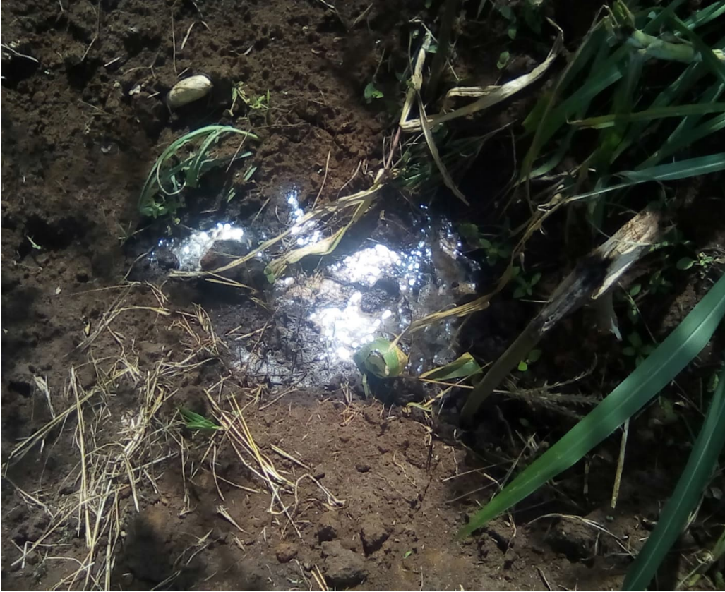
Figure 1 Leakage along the piping
