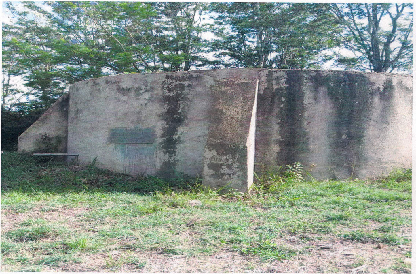
DISTRIBUTION TANK BEFORE REHABILITATION
